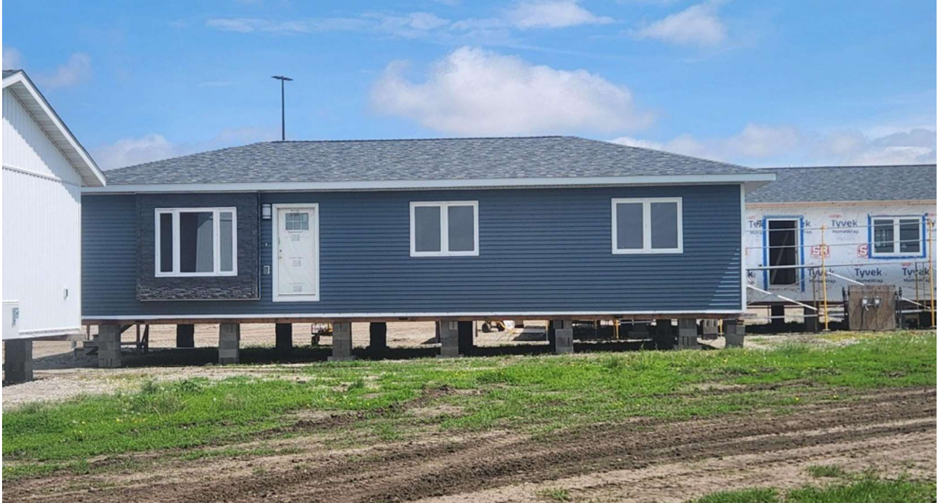
Figure 7: Construction of homes in progress at the Homes for Iowa building site
