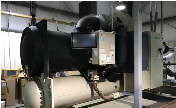
New IVH Chiller
